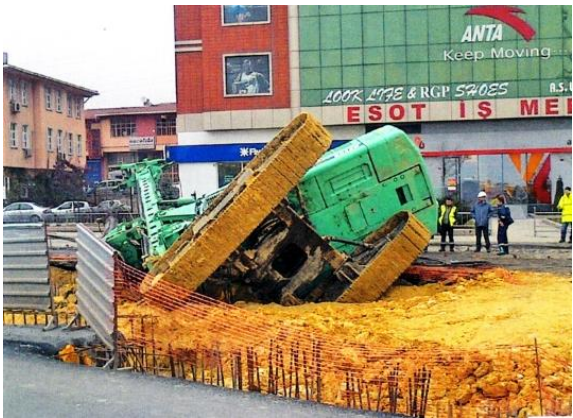
Photo showing failure of working platform and the importance of a safe site
