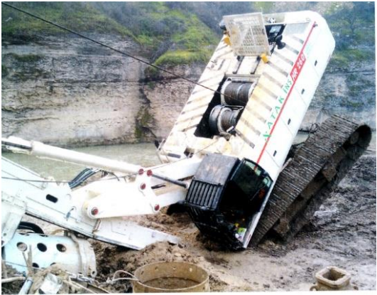
Photo demonstrates the catastrophic consequences of an unsuitable working platform
