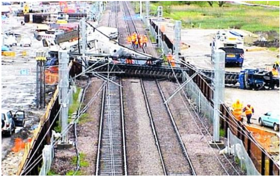
CFA rig collapsed across main London to Paris railway line. Collapse due to improper working platform.
